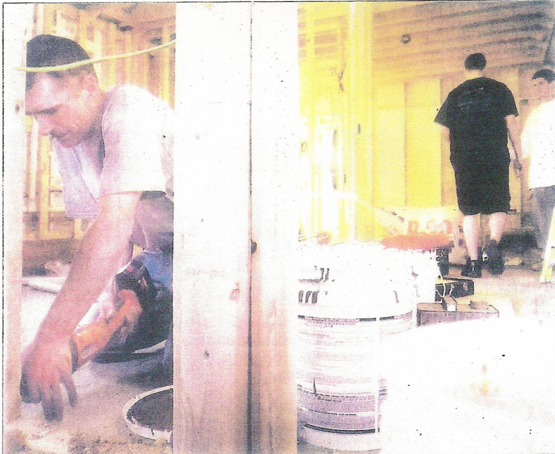
Puro-Tec worker Dan Lynch (left) cuts excess wood out of a door frame as the company works to repair a house in Bristol Township that recently caught on fire. STEVE GEIGLER / STAFF PHOTOGRAPHER
